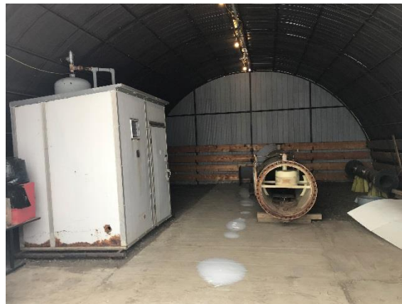
Brias Training Center Indoor Oil Facility
